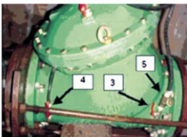
Figura 26 – VRP – controles no manifold
